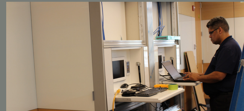
Work in Progress Construction crews and technicians are busy preparing the rooms for the FY17 school year. A technician checks newly-built teaching station to ensure all connections are ready to go.
